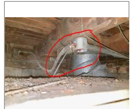
Junction boxes must have a proper cover installed
