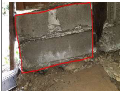
Foundation needs repair on the north side of the house.
