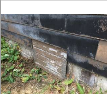
Crawlspace access cover should see all the access .100%.
