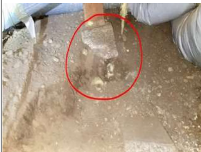
Pier and post need repair.
