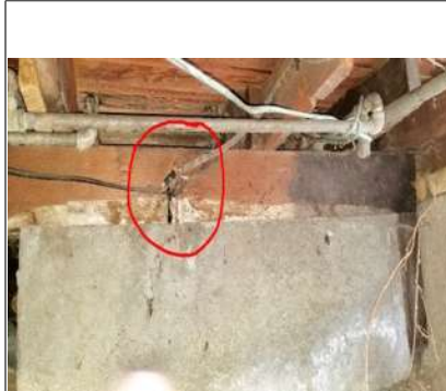
Recommend replacing the wiring in the home.
