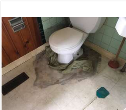
Vinyl flooring and subflooring may need to be replaced.
