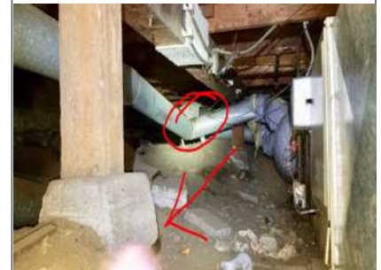
Heating duct needs to be properly supported and insulated,
