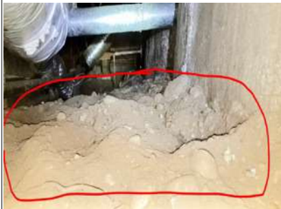
All bare earth in the crawlspace should be covered with a vapor barrier.
