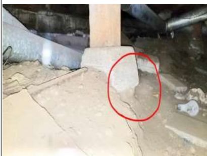
There are a couple of pier and posts systems in the crawlspace that need repair.
