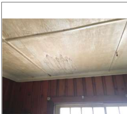
Moisture staining present on the laundry room ceiling.
