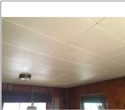
The acoustic ceiling tiles could contain asbestos.
