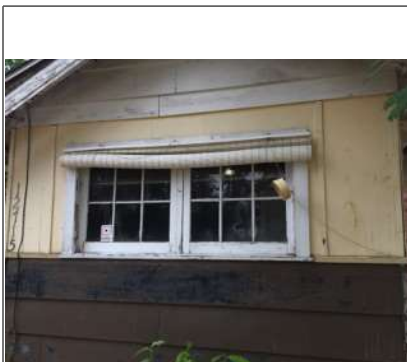
Windows need repair or replacing
