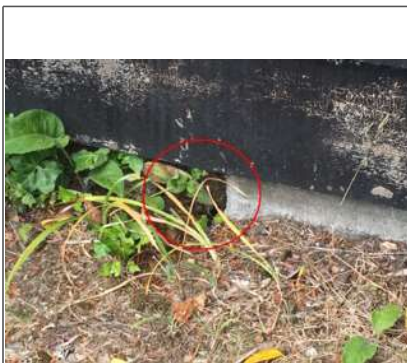
Rotted exposed beam
