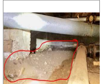
All bare earth in the crawlspace should be covered with a vapor barrier.
