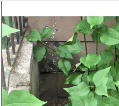
Siding and trim repair. Some of the barge Boards underlayment have damage and may also need to be replaced.
