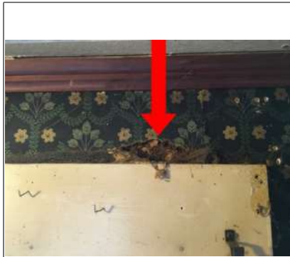
Possibility there is moisture damage wall framing on top of the sliding glass door.
