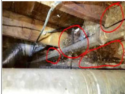
Moisture/insect damaged wall structure and floor joists.
