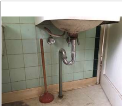
There is no P-trap underneath the sink.
