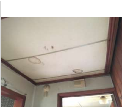
Evidence of moisture intrusion from the attic noted in the hallway.
